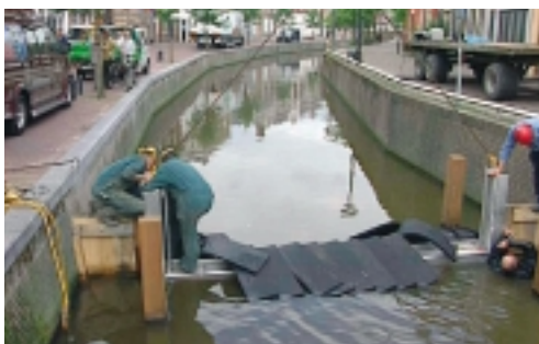
Flexible barrier to separate clean and polluted water, Leeuwarden
