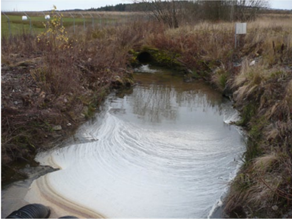
Figure 5: Emergency pond Rovebekken – to be expanded and optimized
