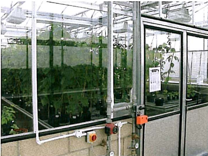
Photograph: Containment cubicles in the high health facility.
