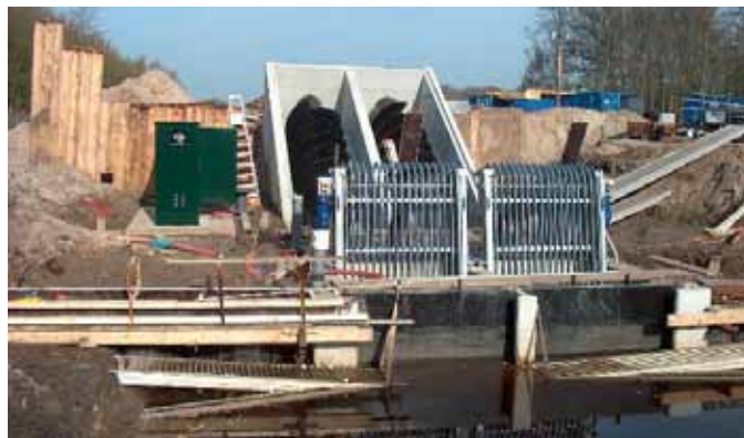
Realisation of fish friendly pumping station Ennemaborgh
