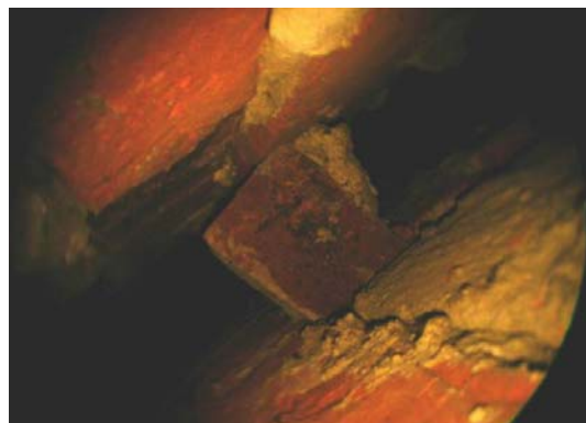
Endoscope image → in the area where a defect was suspected there is, indeed, no insulation!
