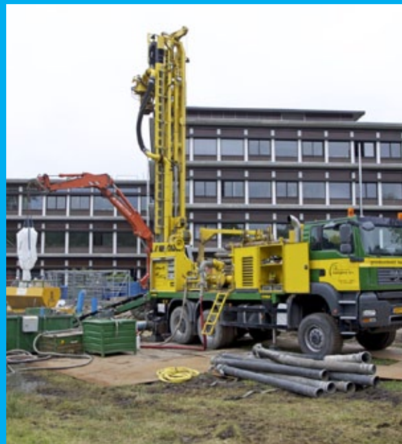
Construction works at the Provinciehuis - the thermal storage system.
