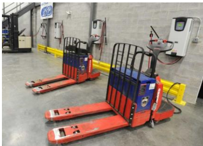
Figure 3 – Charging point for electric forklift 1 .
