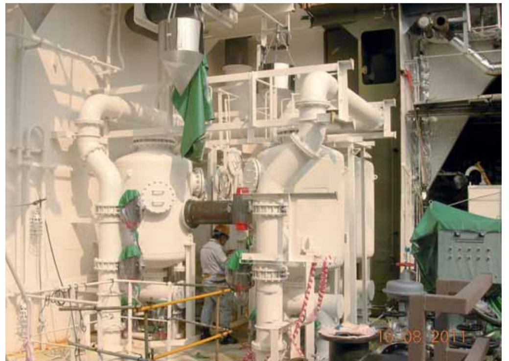
IMO Type Approved BWM System 2500 m 3 /hr capacity installed in a tanker pump room. Photo compliments of Hyde Marine
