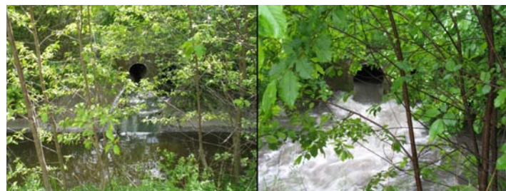
Comparison of a waste water outlet at the Danish case study under both, dry (left) and intensive rain (right) weather conditions.
